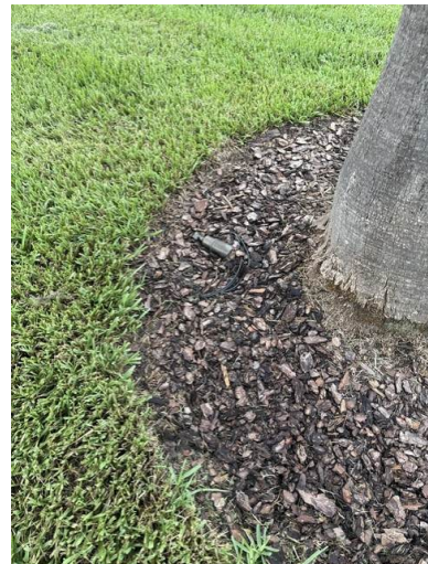
Displaced fixture and damaged mounting stake.
