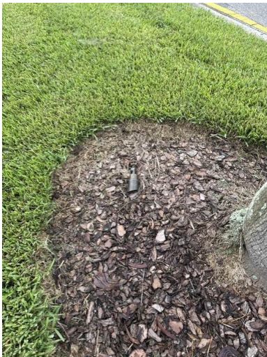
Fixture knocked down at a rear center-median palm.
