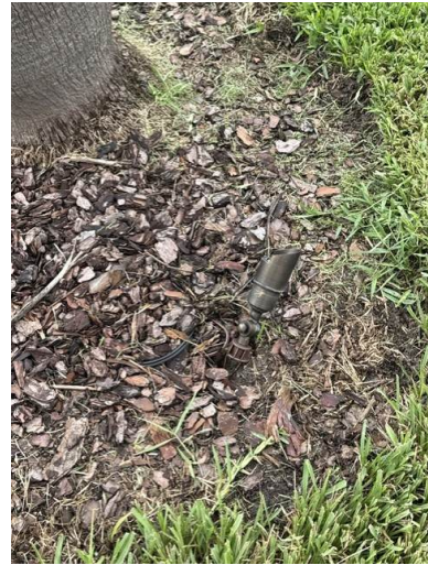
Close view of the physically damaged fixture assembly.
